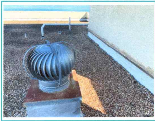
13 Additional areas of subsurface water along N. end Elev.
