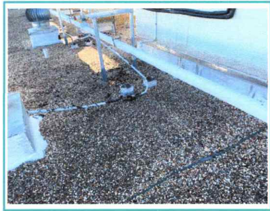
14 Subsurface water detected at base of Elev. Hs. & stands
