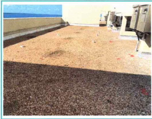
9. Large area of high concentration subsurface water, wet
