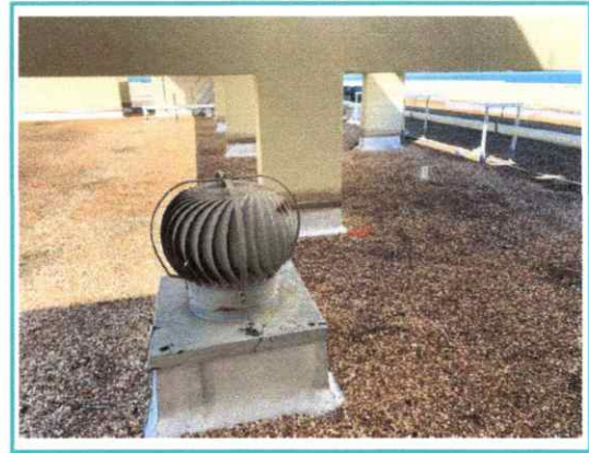
12. Subsurface water continues within center of roof, wet
