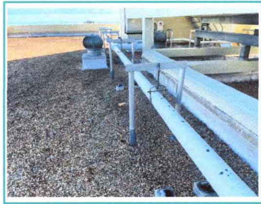
16 Subsurface water continues surrounding pipe stands
