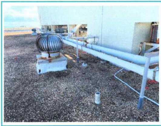
15 Subsurface water detected at base of Elev. Hs. & stands
