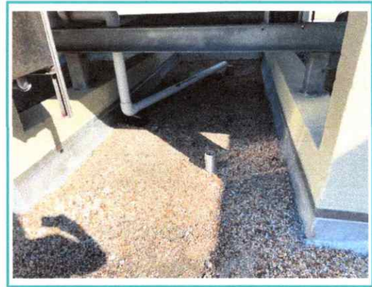
10. Additional areas of subsurface water under C. Twr.
