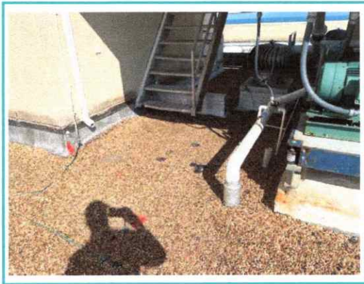
11. Additional areas of subsurface water under C. Twr.
